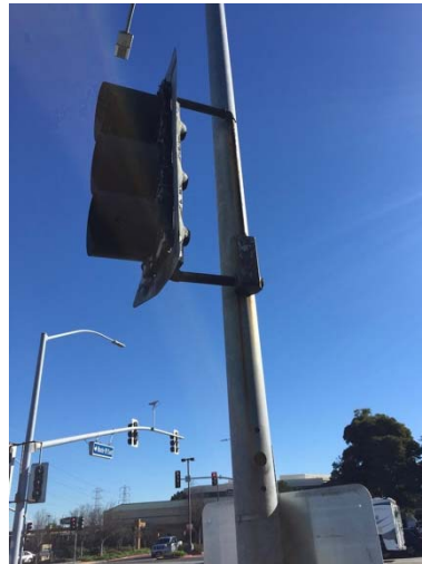
Oxidized Pedestrian Push Buttons and Traffic Signal Framework.
